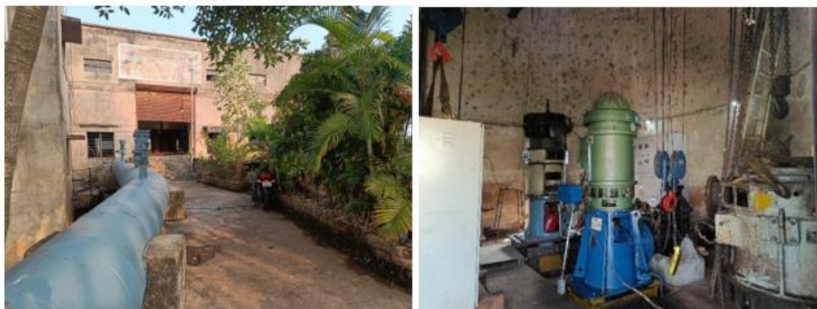
Figure 4-1 Photographs of Majarewadi and Panchganga Pumping Station
